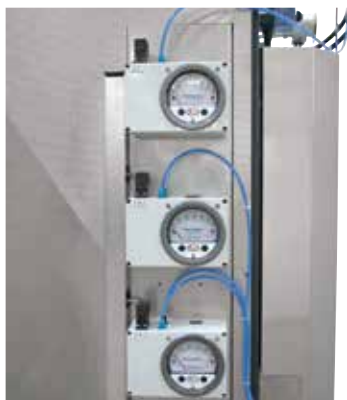
Pressure and flow rate displayed as part of debinding package II
