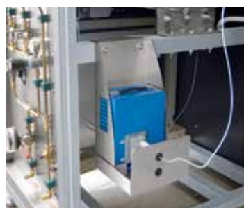
Acid pump for nitric acid
