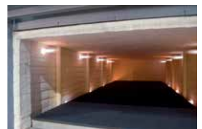
Furnace chamber with eight high-speed burners
